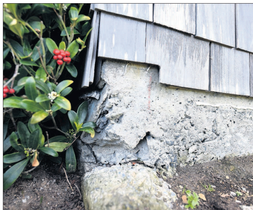
Damage can be seen to the foundation of City Hall in Cannon Beach.
