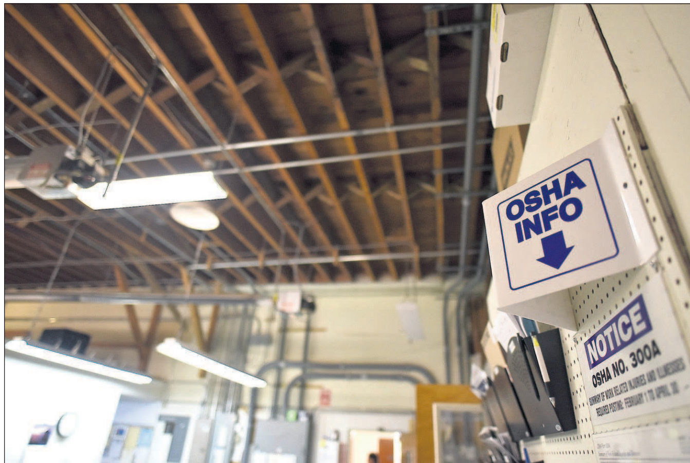
The ceiling at Cannon Beach City Hall has been known to leak.
