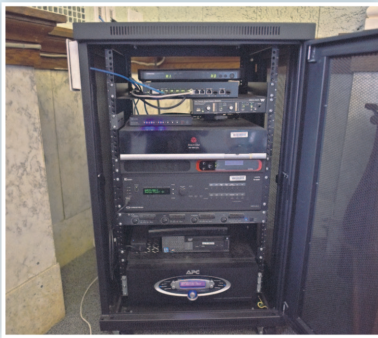
Recording equipment in a cabinet in courtroom 300 at the Clatsop County Courthouse.
