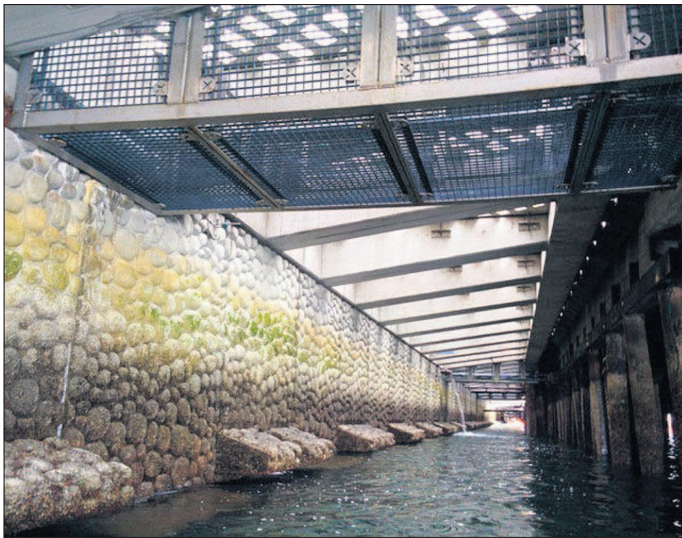
A view of the new seawall being installed on the Seattle waterfront. It's designed to help juvenile salmon.
