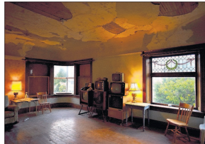
Colin Murphey/The Daily Astorian The interior of the George C. Flavel home is nearly ready for the final touches of the restoration process.
