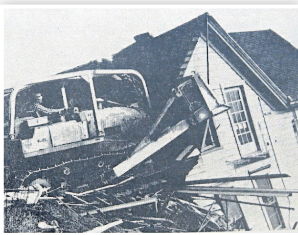
1968 — This bulldozer, operated by Art McCoy, pushed the house at 10th and Grand over the bank this morning and demolished it. The ground there will be cut down and used to extend an apartment project.
