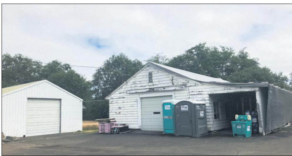
Some of Clatsop Community College's maritime classes are held in a deteriorating U.S. Army Corps of Engineers building next to campus. The college is hoping to modernize its maritime programs.
