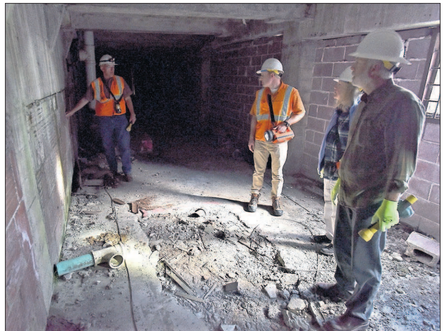
Astoria city leaders toured a section of tunnel in October next to the pit.
