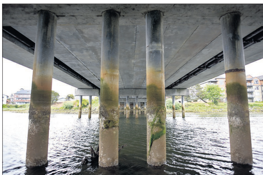
Multiple bridges and roads in Seaside have been deemed problematic during a recent study of the effects of an earthquake and tsunami in the area.
