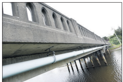
One of the bridges over 12th Street in Seaside is an example of infrastructure in the area that could fail in an earthquake.
