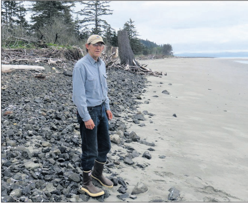
David Cottrell stands on an example of dynamic revetment protecting shoreline from further erosion at Washaway Beach.
