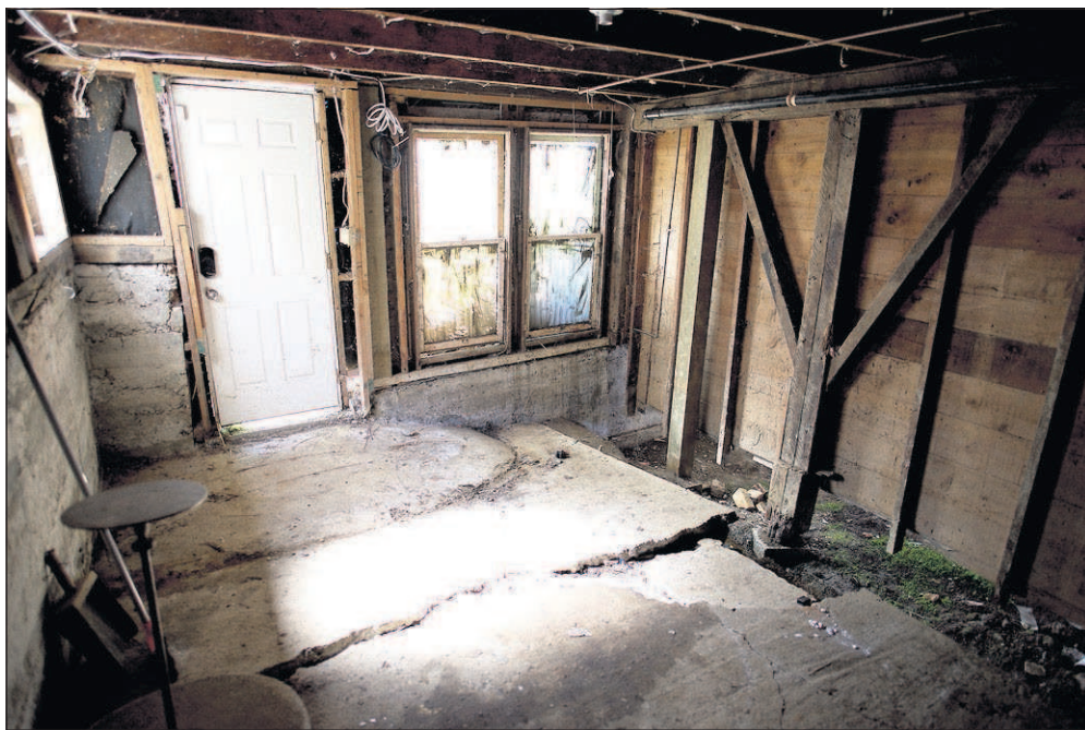
The basement of the house on Alameda Street shows signs of structural issues.
