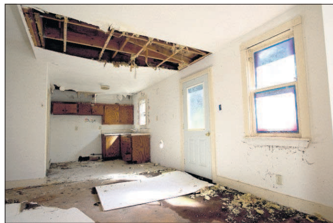
The interior of the property shows signs of damage and decay.
