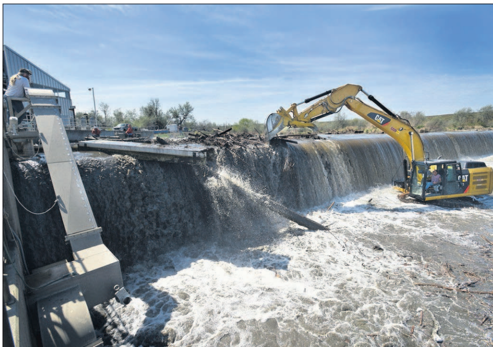
An excavator and a motorboat are used to break a log jam in April 2013 above the Three Mile Dam on the Umatilla River north of Hermiston.
