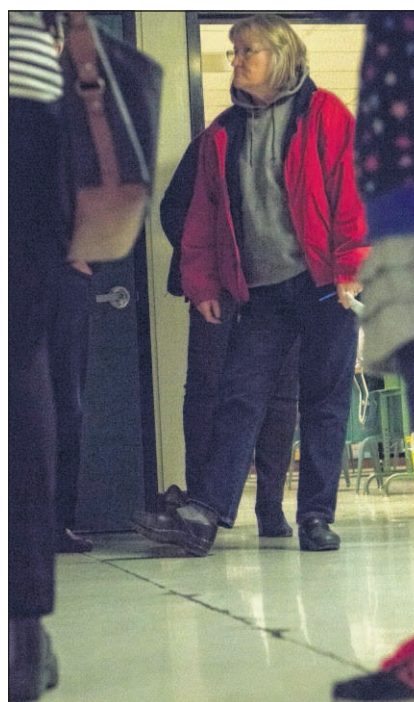
Although structurally sound, Astoria Middle School faces cracks in its floors.
