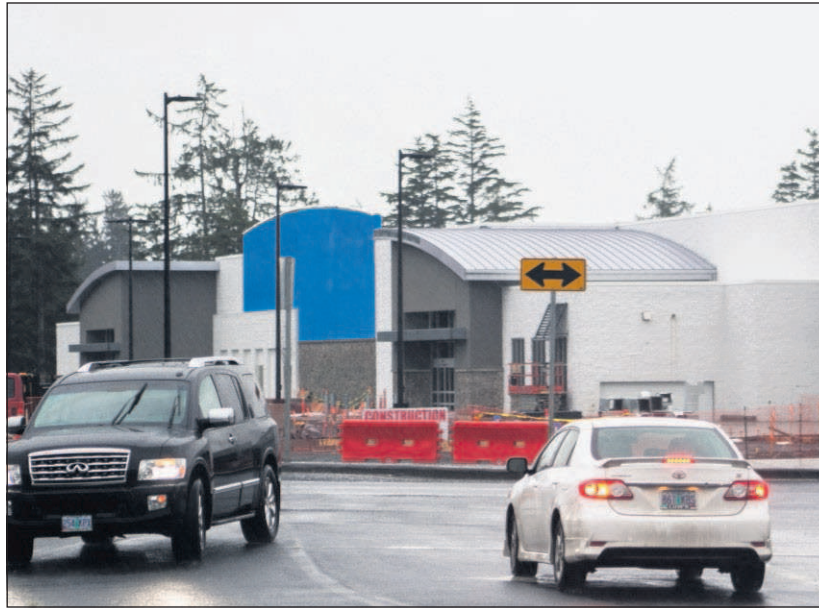
The new Walmart Supercenter under construction at the North Coast Retail Center in Warrenton will open June 13.
