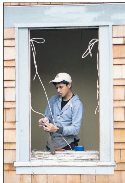
Jose Luis Roidan Perez, a first-year historic preservation and restoration student at Clatsop Community College, fixes a rope pulley system in a window at Astoria's Alderbrook Hall.
