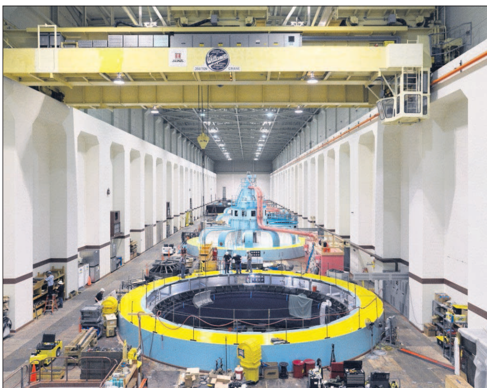
An overhead crane is used to remove a piece of main unit power generator in 2014 at McNary Dam on the Columbia River outside of Umatilla.
