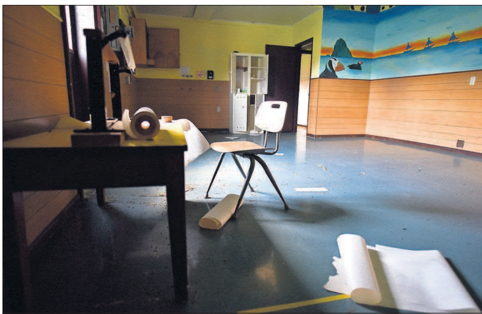
Signs that students once occupied classrooms remain four years after the Cannon Beach Elementary School shut down.
