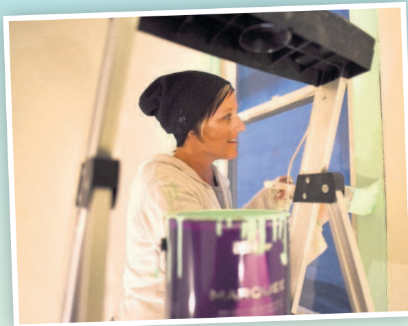
Lucy Barna puts a fresh coat of paint on a window sill in the Van Dusen Building in Astoria.
