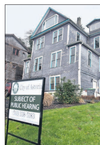
Colin Murphey/The Daily Astorian A house on Alameda Street in Astoria is the subject of a preservation debate.
