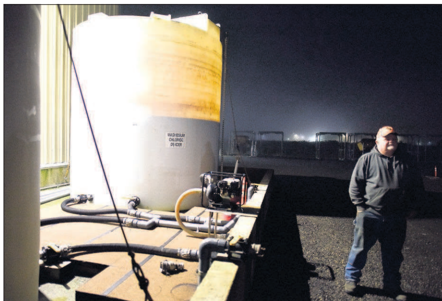
Wade Tucker stands next to a tank of magnesium chloride, which is used by the Oregon Department of Transportation to treat area roads for ice.
