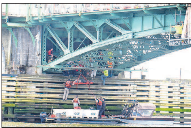
Colin Murphey/The Daily Astorian Purcell Painting & Coatings employee Merle Hicks suffered serious injuries after falling off a mobile scaffolding system while working on the Old Youngs Bay Bridge.
