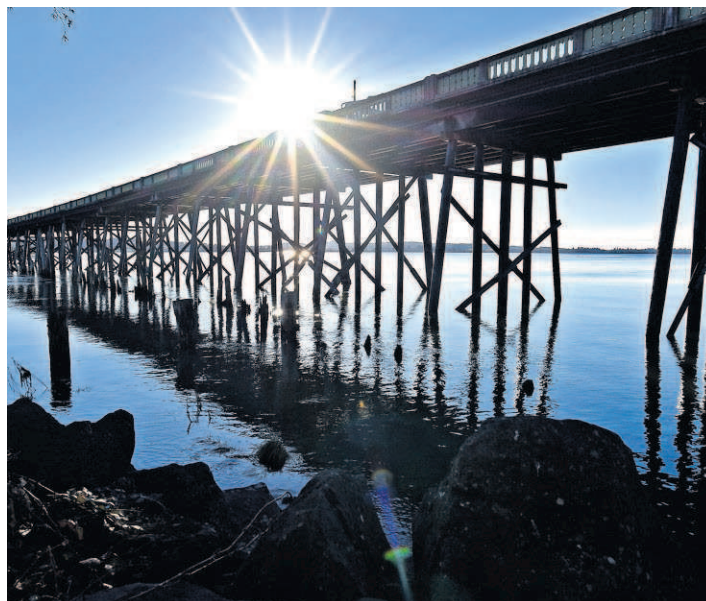
Work to repair the Old Youngs Bay Bridge was completed earlier this year.
