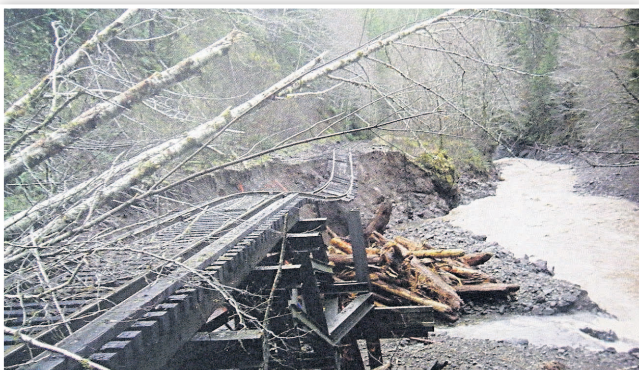
The Port of Tillamook Railroad suffered some of the most visible damage from the storm that hit Dec. 2 and 3. Tracks here buckled as support ground was washed away.
