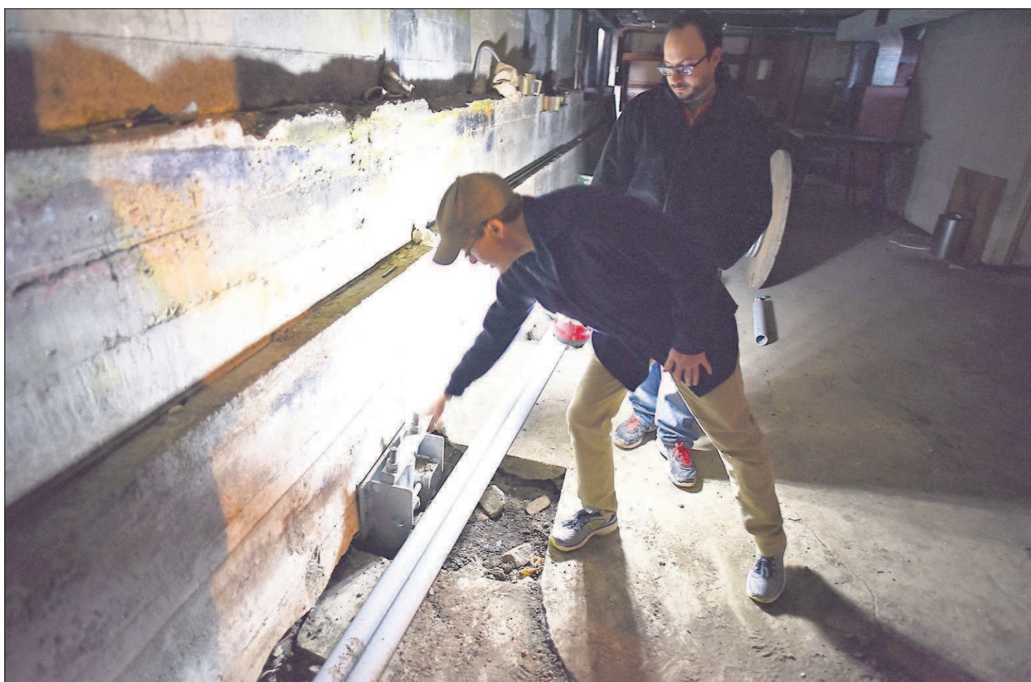
John Goodenberger, a local expert in historic buildings, points out earth anchors installed in the basement.
