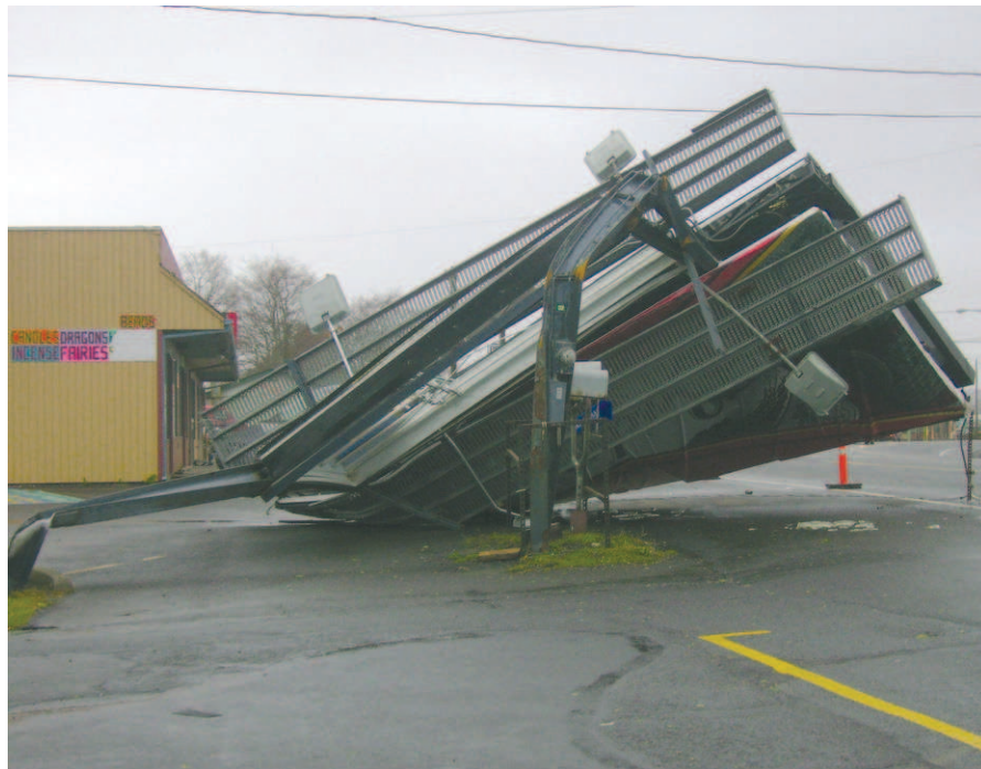
A business sustained damage in high winds.
