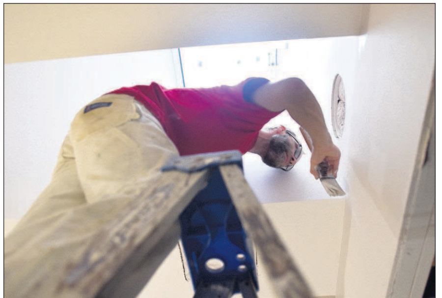
Aaron Olson paints the ceiling of a new home in Cannon Beach for Coaster Construction.
