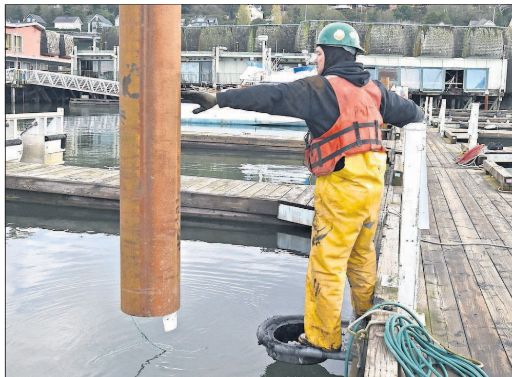
A replacement piling is lowered into place Monday at the Port of Astoria's West End Mooring Basin.
