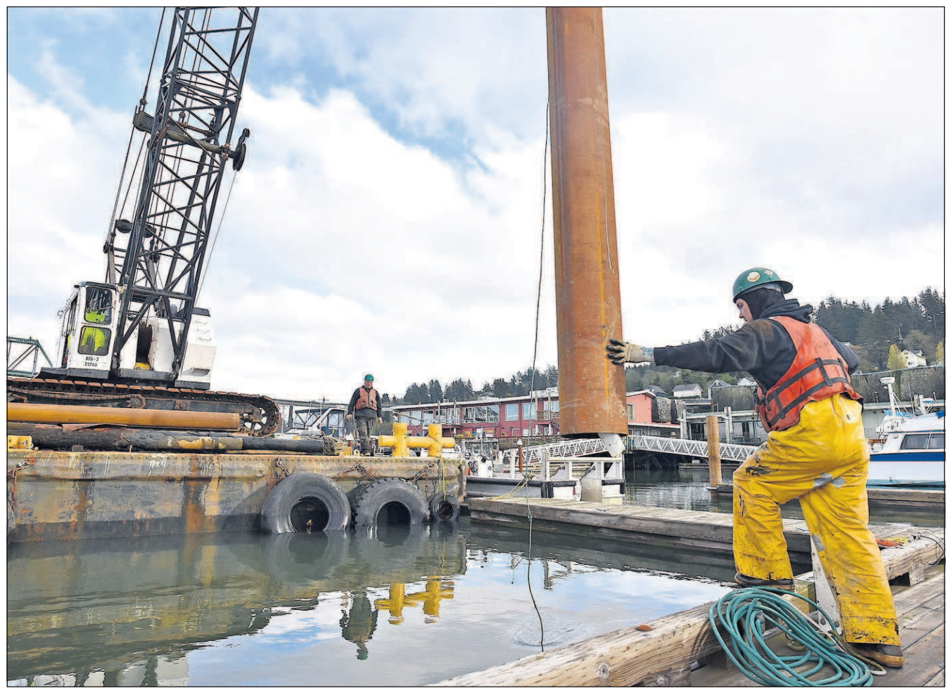
Pilings are replaced Monday at the West End Mooring Basin while elsewhere at the facility, a routine dredging operation was underway.
