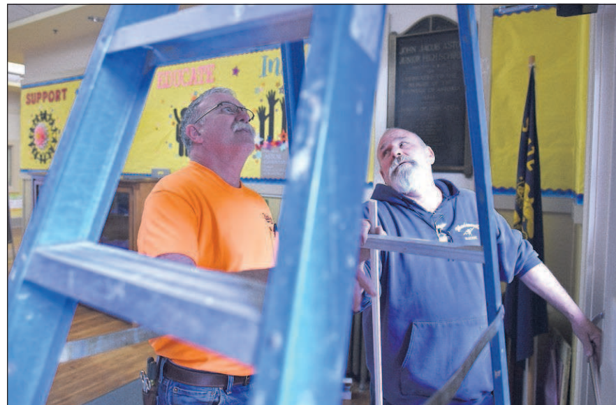
John Moeller, left, and Jack Dickey work to install new security measures at Astor Elementary School in Astoria.
