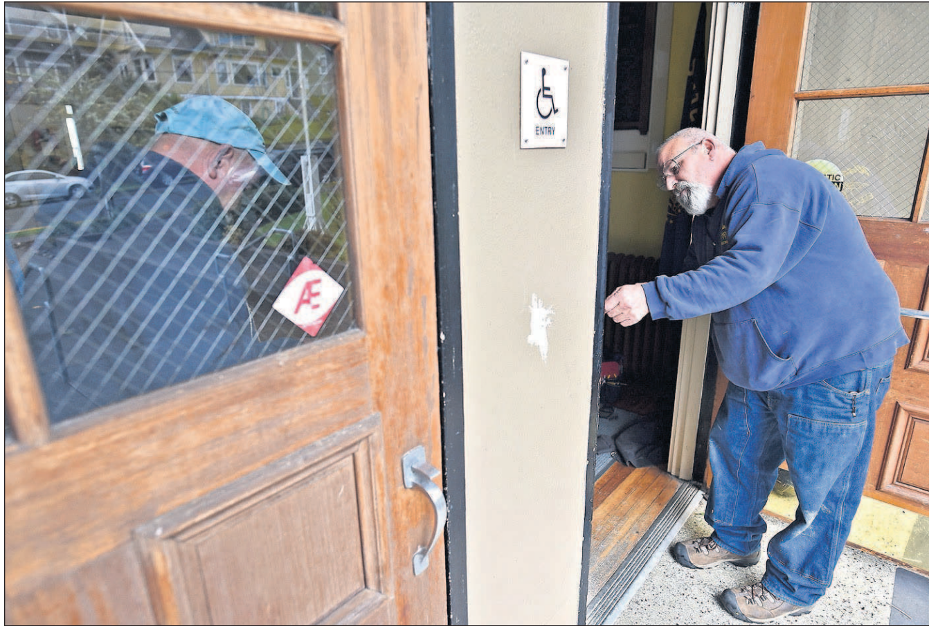
Mike Rath, left, and Jack Dickey prepare the front entrance of Astor Elementary School in Astoria for new security measures.
