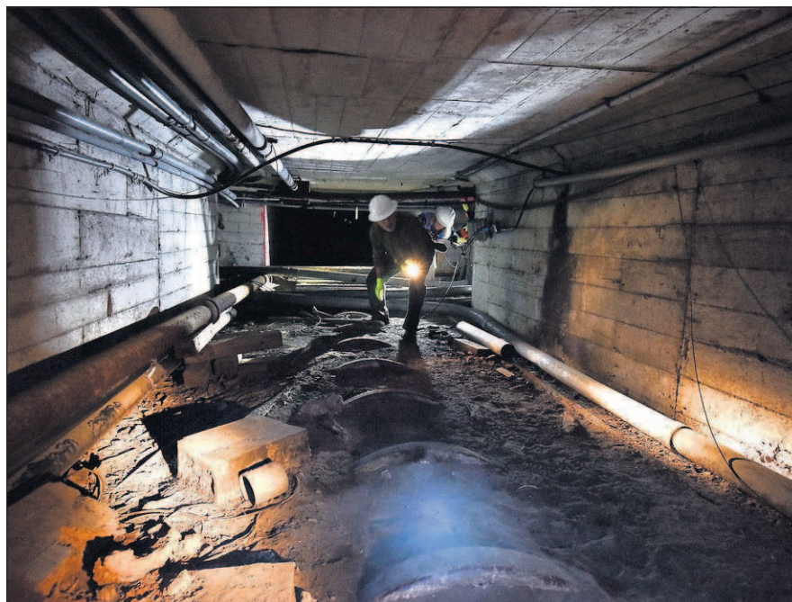
Astoria city councilors make their way through a small system of tunnels under the city during a recent informational tour.
