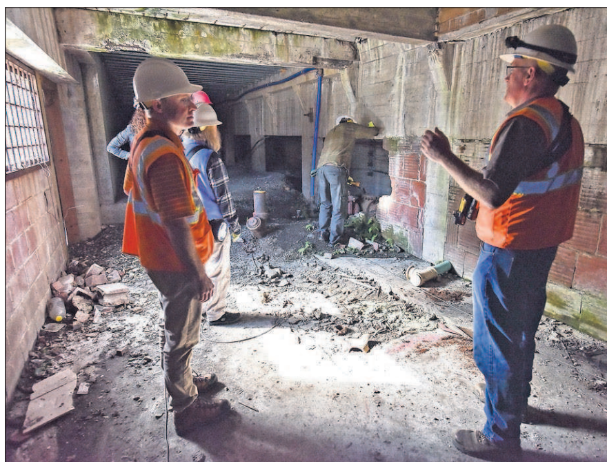
Astoria Assistant City Engineer Nathan Crater, left, and Public Works Superintendent Ken Nelson, right, lead a group of city officials on a tour of a section of tunnels under the streets of Astoria.
