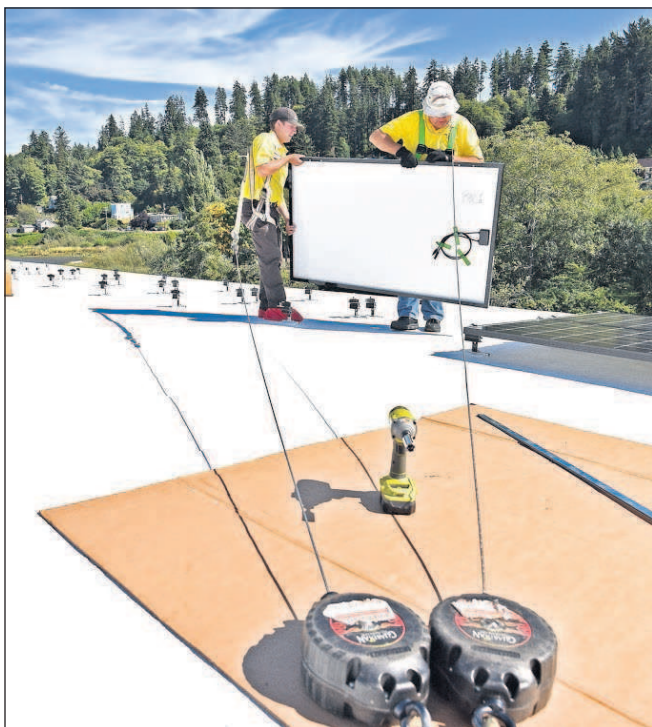
Eddie Phillips, left, and Chuck Waddell, right, with Precision Heating and Indoor Air Quality of Warrenton secure themselves to the roof of Alderbrook Station in Astoria as they install solar panels for a client.
