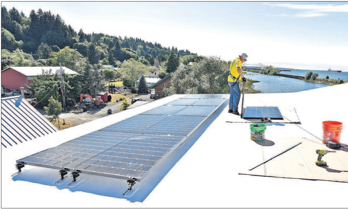
Chuck Waddell gets ready to install one of 34 solar panels on the roof of Alderbrook Station in Astoria in late August. According to City Planner Nancy Ferber, the city sees few applications for similar projects.
