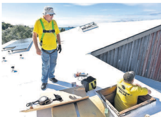
Workers with Precision Heating and Indoor Air Quality of Warrenton recently installed an array of 34 solar panels on the roof of Alderbrook Station in Astoria. More photos at DailyAstorian.com
