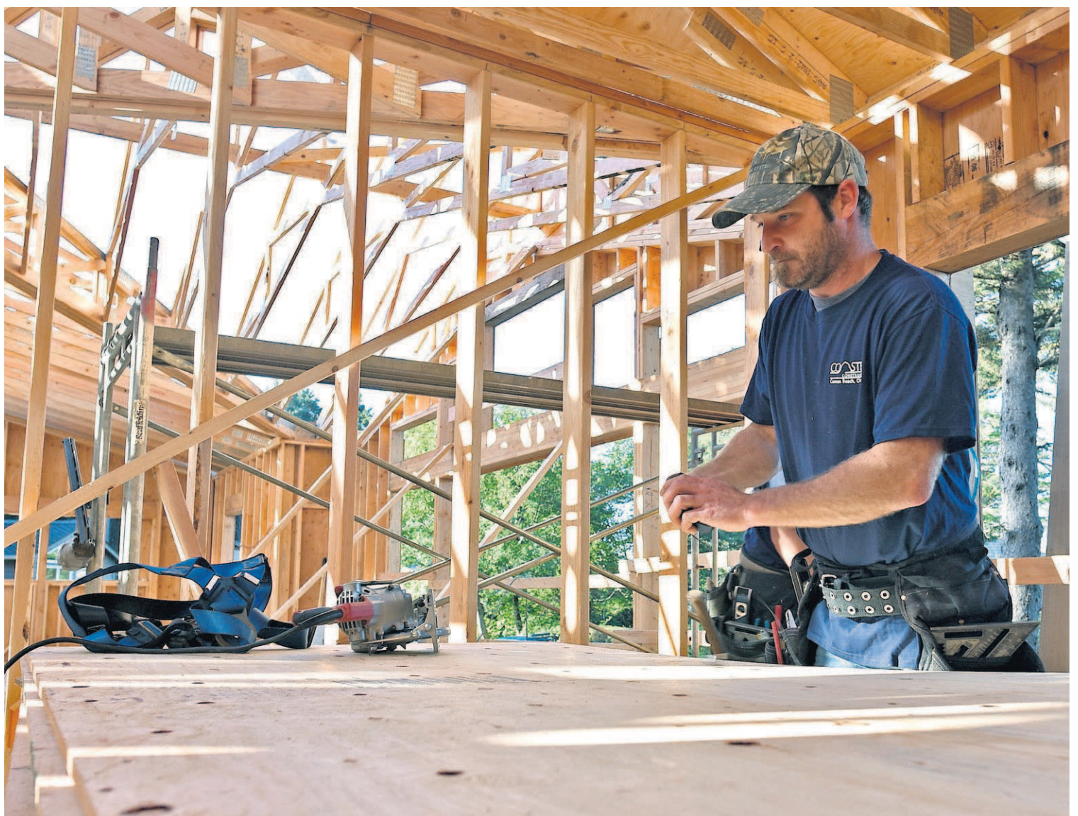
Chris Erickson of Coaster Construction prepares to measure a sheet of plywood at one of the sites of new home construction in Cannon Beach.
