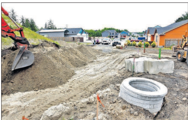
Utility construction continues on the northern extension of the Juniper Ridge subdivision in Warrenton.
