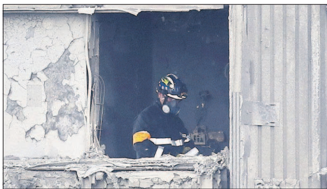
Rick Findler/PA Fire service personnel are inside Grenfell Tower today in west London after a fire engulfed the 24-story building Wednesday morning. A London fire commissioner says it will take weeks for the building to be searched and cleared.
