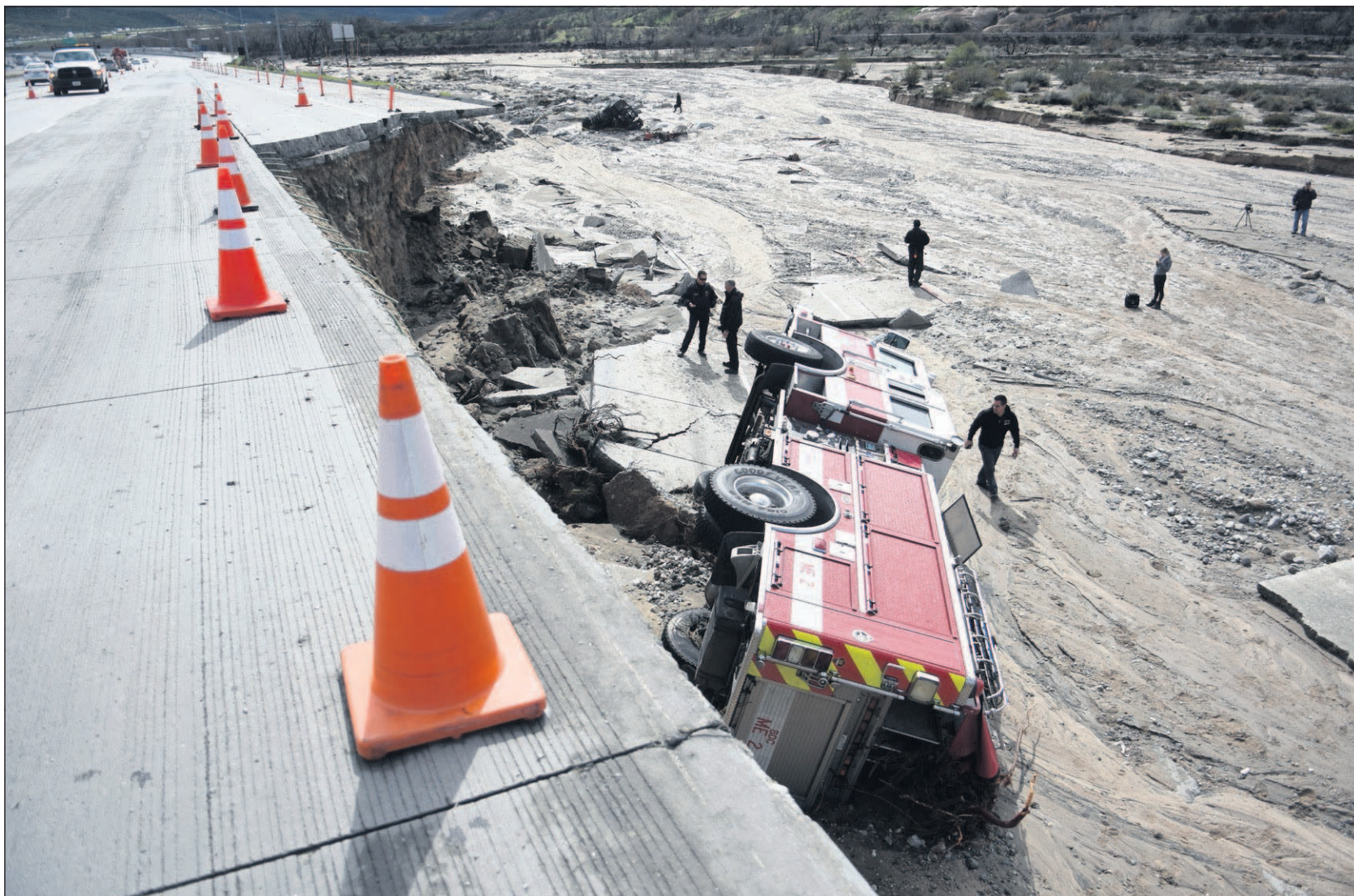
Officials look over the scene at Interstate 15 in the Cajon Pass, Calif., where part of the freeway collapsed due to heavy rain in February. David Pardo/The Daily Press
