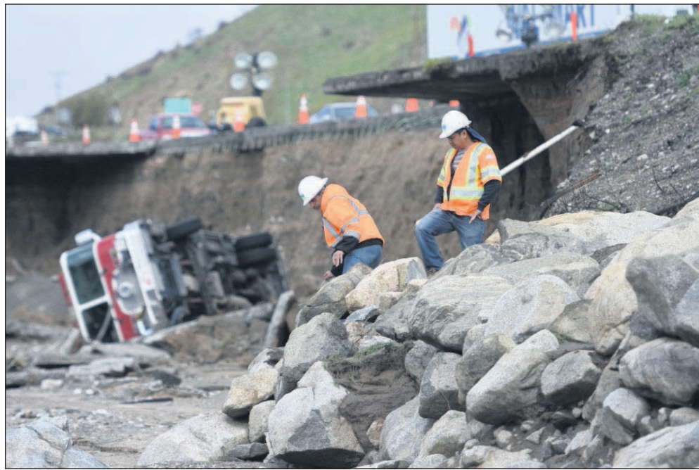
Crews look over a tractor trailer and a San Bernardino County Fire Department fire engine that fell from southbound Interstate 15 where part of the freeway collapsed due to heavy rain in the Cajon Pass, Calif., in February. David Pardo/The Daily Press
