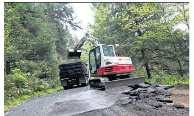
Colin Murphey/The Daily Astorian Heavy construction equipment was brought to Ecola State Park last week to repair damage from a series of landslides that occurred in multiple locations in the park.
