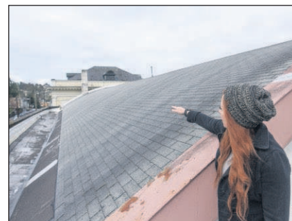
Danny Miller/The Daily Astorian Astoria Armory Executive Director Robyn Koustik points to a section of the Armory roof that was damaged during a windstorm on Friday in Astoria.
