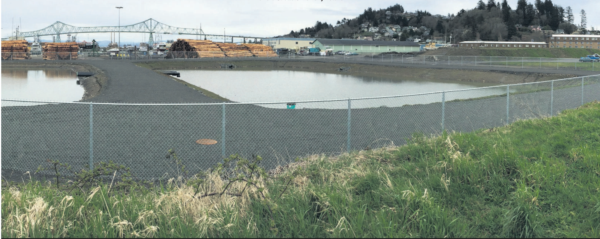
Port of Astoria Executive Director Jim Knight said there are issues with a berm surrounding the retention ponds delaying completion of the agency's new stormwater treatment system on Pier 3. Edward Stratton/The Daily Astorian
