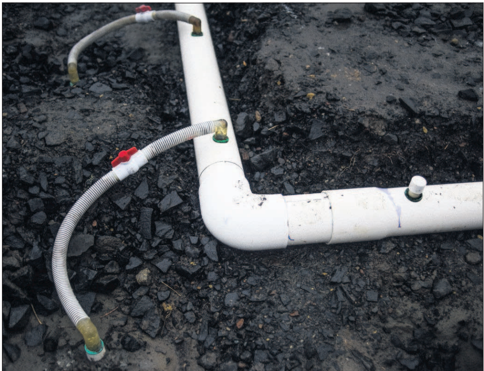
Danny Miller/The Daily Astorian Construction continues on a new pump station on Wednesday in Warrenton.
