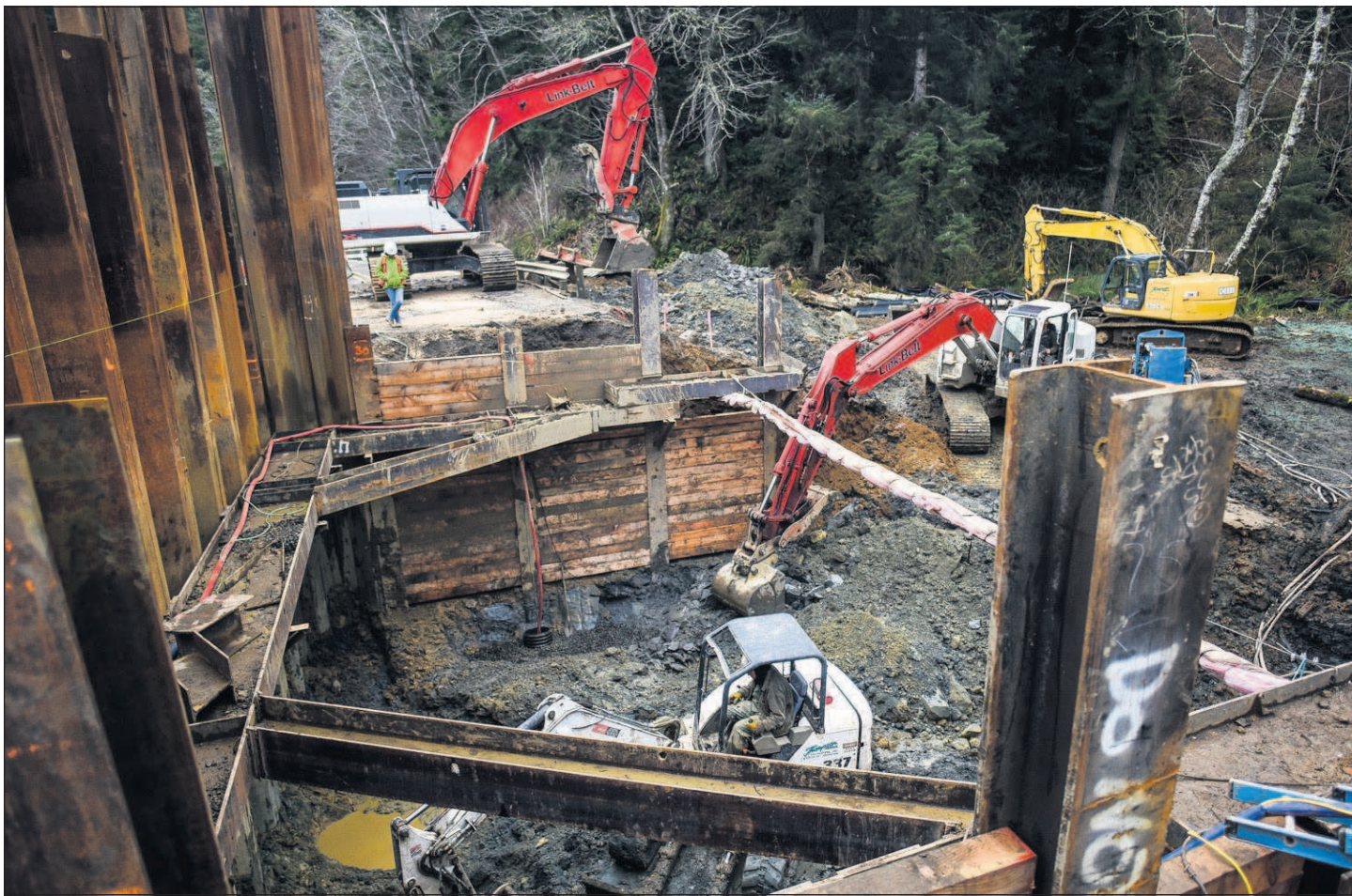
Danny Miller/The Daily Astorian A crew works on CREST's Columbia-Pacific Passage Habitat Restoration project located along Highway 401 on Thursday in Washington.
