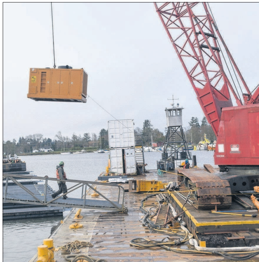
Bergerson Construction workers load a vibratory hammer onto a barge in order to continue work on a new dock Monday at the Warrenton Marina.
