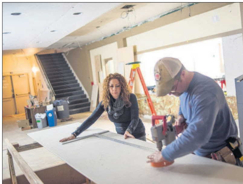
Robyn Kous-tik, director of the Astoria Armory, left, works with volunteers from the U.S. Coast Guard, Bogh Electric, and JP Plumbing who are helping to remodel the lobby space in the Armory on Thursday.
