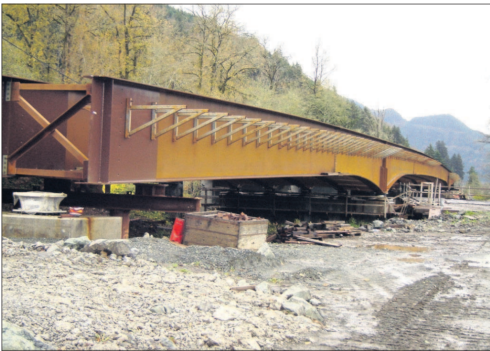
With the steel framework now in place the new Lommen Bridge, which spans the Nehalem River on Miami-Foley Road in north Tillamook County, is beginning to take shape. Dave Fisher/For EO Media Group
