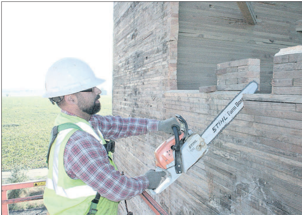
Darell Braman of Northwest Reclaimed Wood, a deconstruction company, dismantles a grain elevator in Suver. Old wood from barns and other farm buildings is popular among woodworkers and home renovators.
