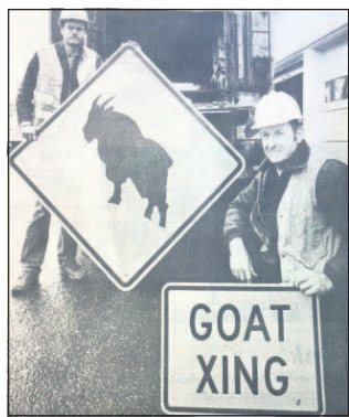
The News-Review In this undated photo, state highway workers install goat crossing signs on Interstate 5 in Roseburg.
