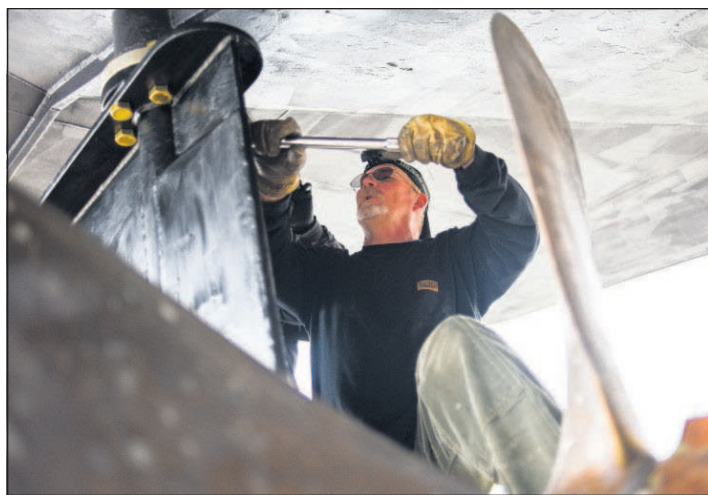
J&H employee Kevin Eaton works to install a replacement rudder on the Taasinge.
