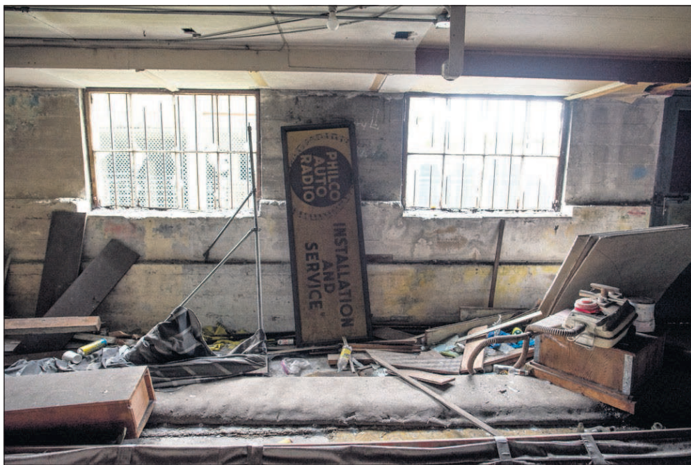
Leftover debris litters the floor in the basement of the M&amp;N Building.
