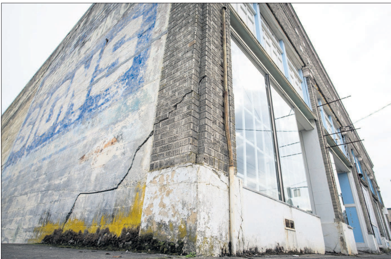
A crack in the M&amp;N Building is visible from Ninth Street.
