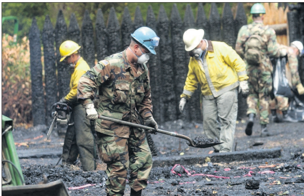
National Guardsman and others work to clean up after the 2005 fire at Fort Clatsop.
