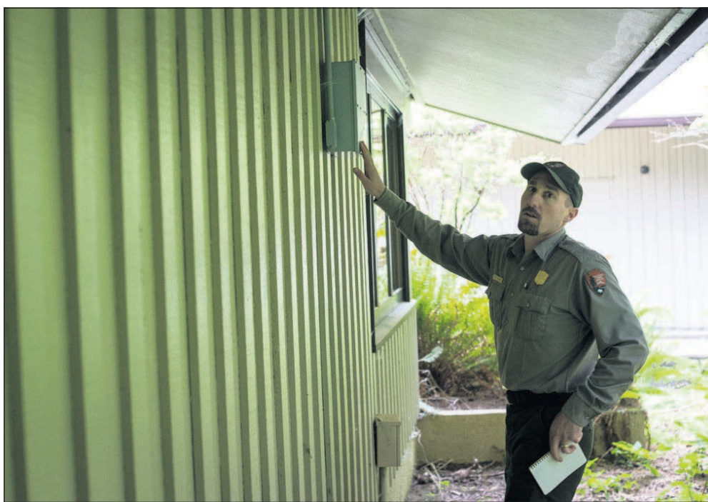
Joshua Bessex/The Daily Astorian Matt Shaefer, the park’s chief of facility management, stands near a receiver that works as part of the park’s fire-alarm system.
