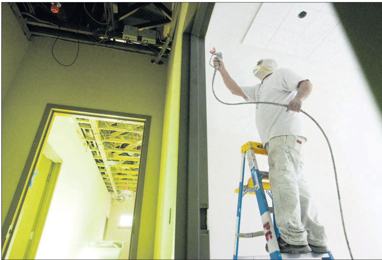
Daric Williams paints one of the probation offices in the new Clatsop County Sheriff's Office on Wednesday. Joshua Bessex/The Daily Astorian
