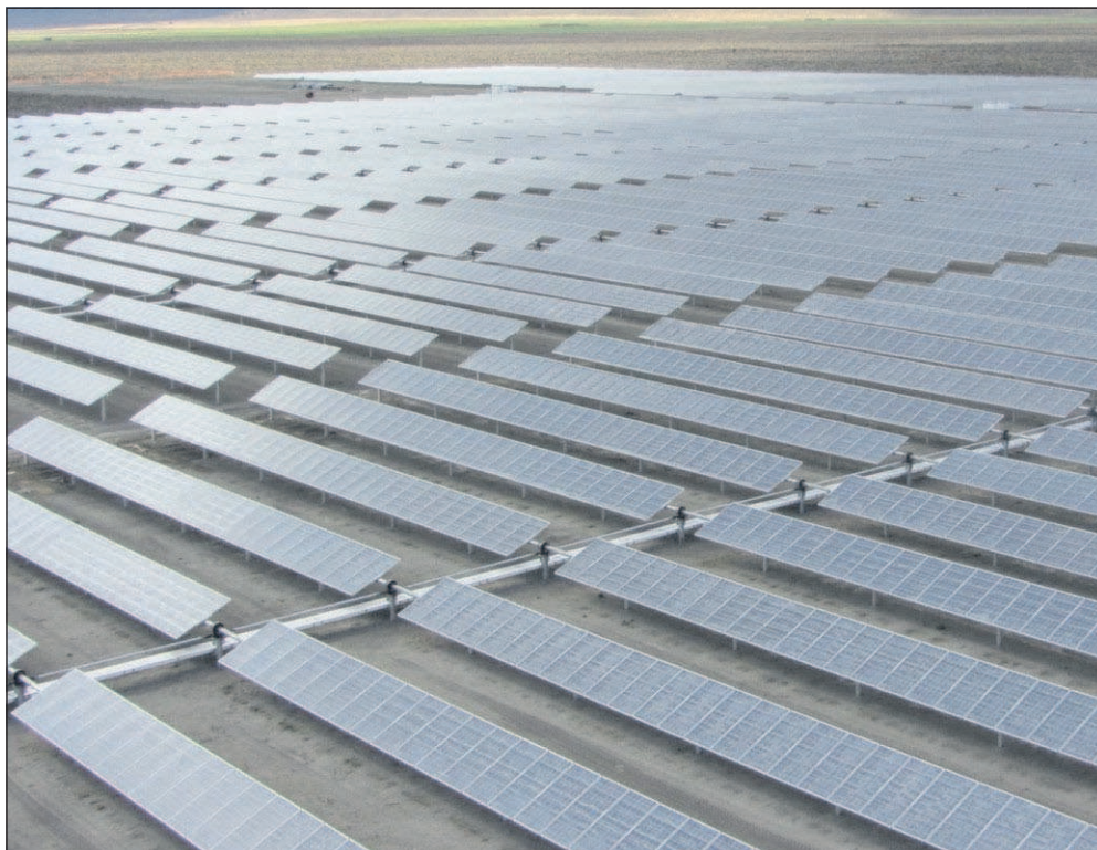
The Outback project in southern Oregon, east of Christmas Valley. The five-megawatt project provides power for Portland General Electric.
