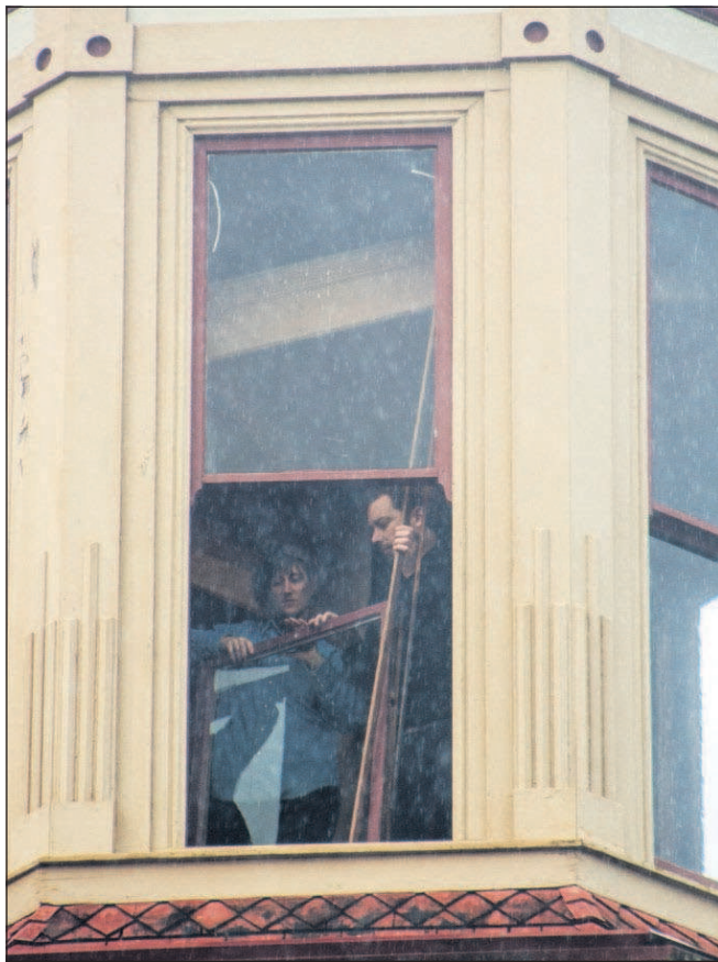
Students in Clatsop Community College historic preservation and restoration program popped out the historic sash windows on the upper turret of the Flavel House Museum during a hands-on workshop over the weekend.
